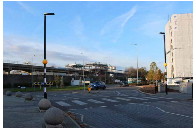
View of Brunel Roundabout with transfer building for East West Rail under construction
